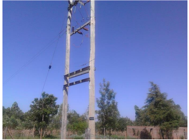
Transformer not found on ground
