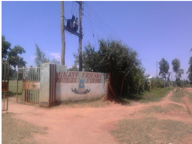
Transformer at Mikayu Friends Primary School
