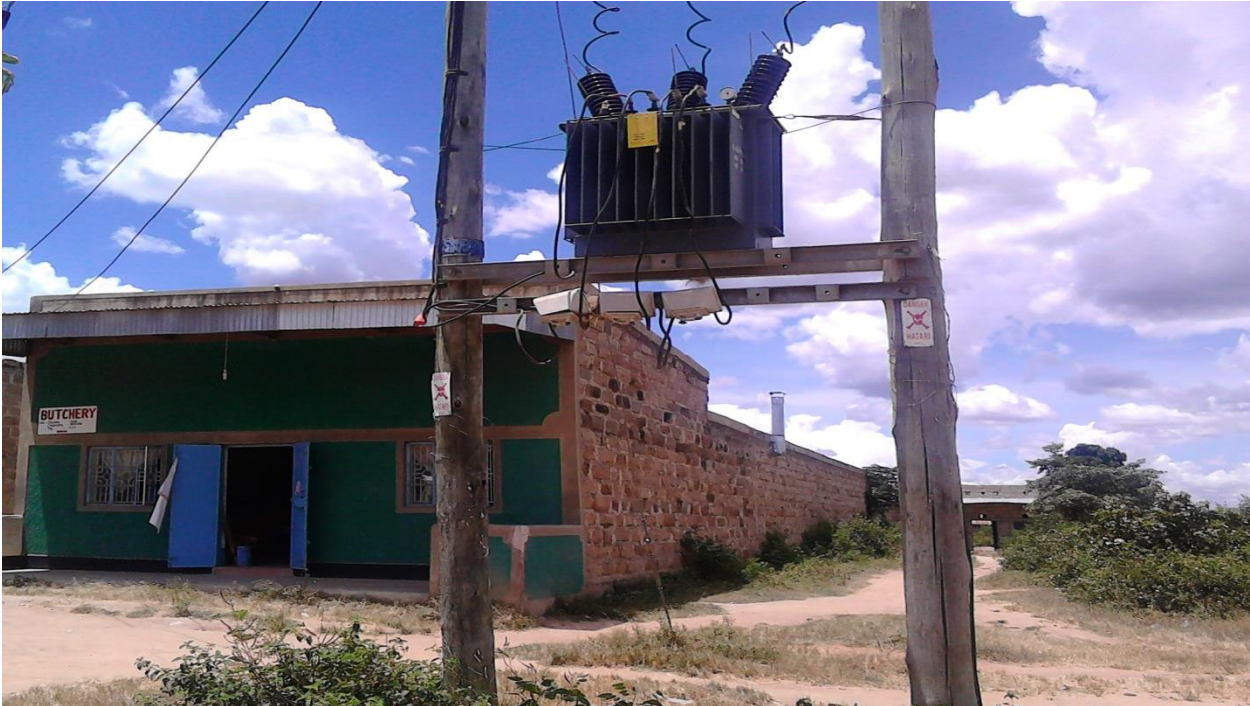
One of the transformers in Machakos County
