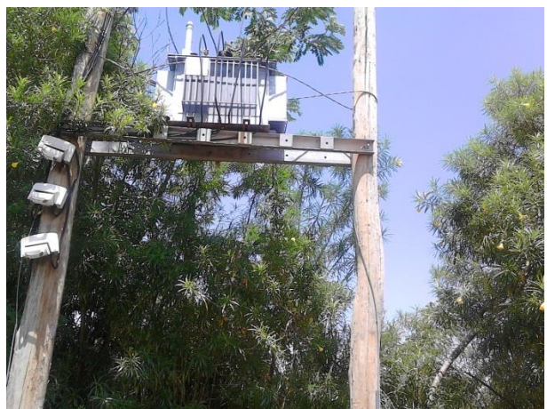
Transformer number not marked on ground
