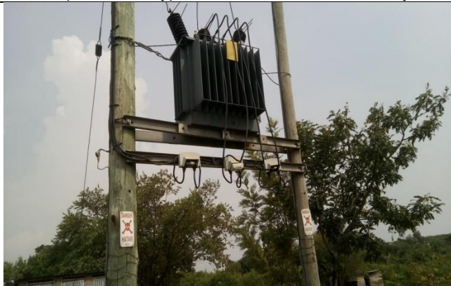
A sample of the transformer to be maximized
