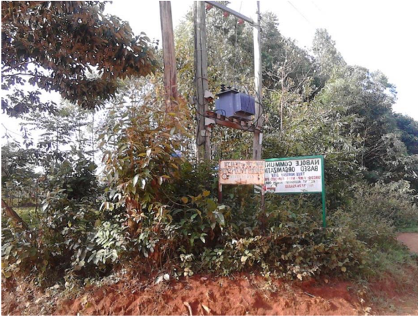
Way leave maintenance required on 11 kV powerline from Nabola Transformer
