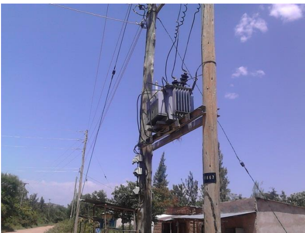
Transformer number 41867 on ground
