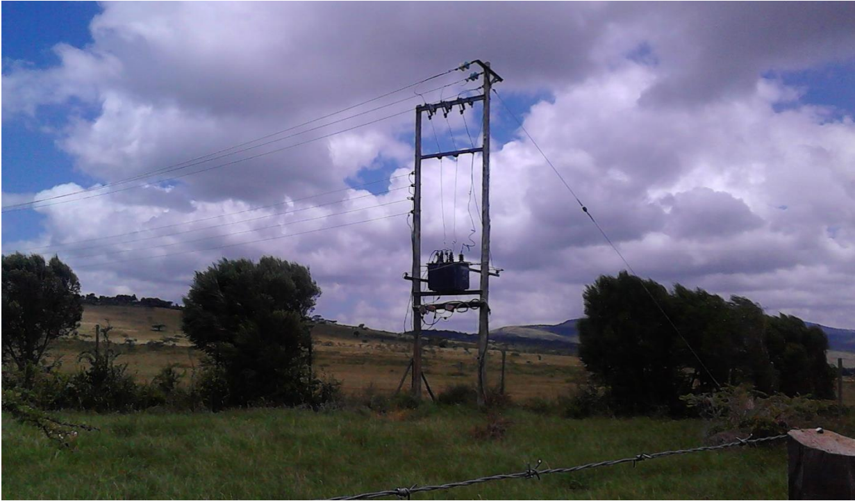
One of the transformers in Kajiado County with its surrounding environment
